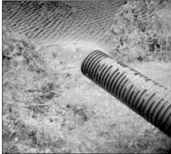
This poorly installed road drainage outfall demonstrates the direct link between streets and streams. © TRK
